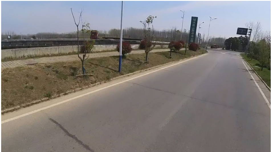
纵横向裂缝、侧石及雨水算子破损
