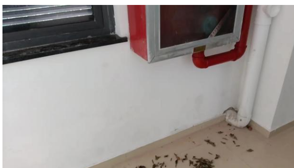
一楼走廊墙面渗漏
